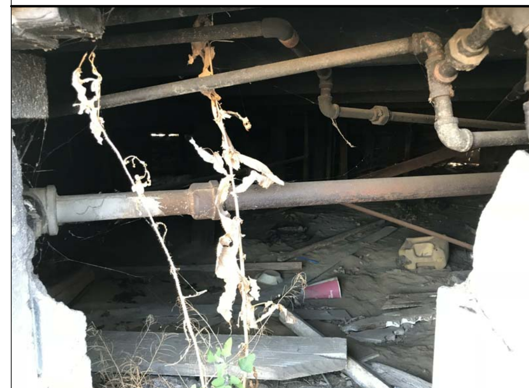
ALL FIRE DAMAGE WATER LINES OR IT DOES NOT MEET CBC 2016 WILL BE REMOVED AND REPLACED
