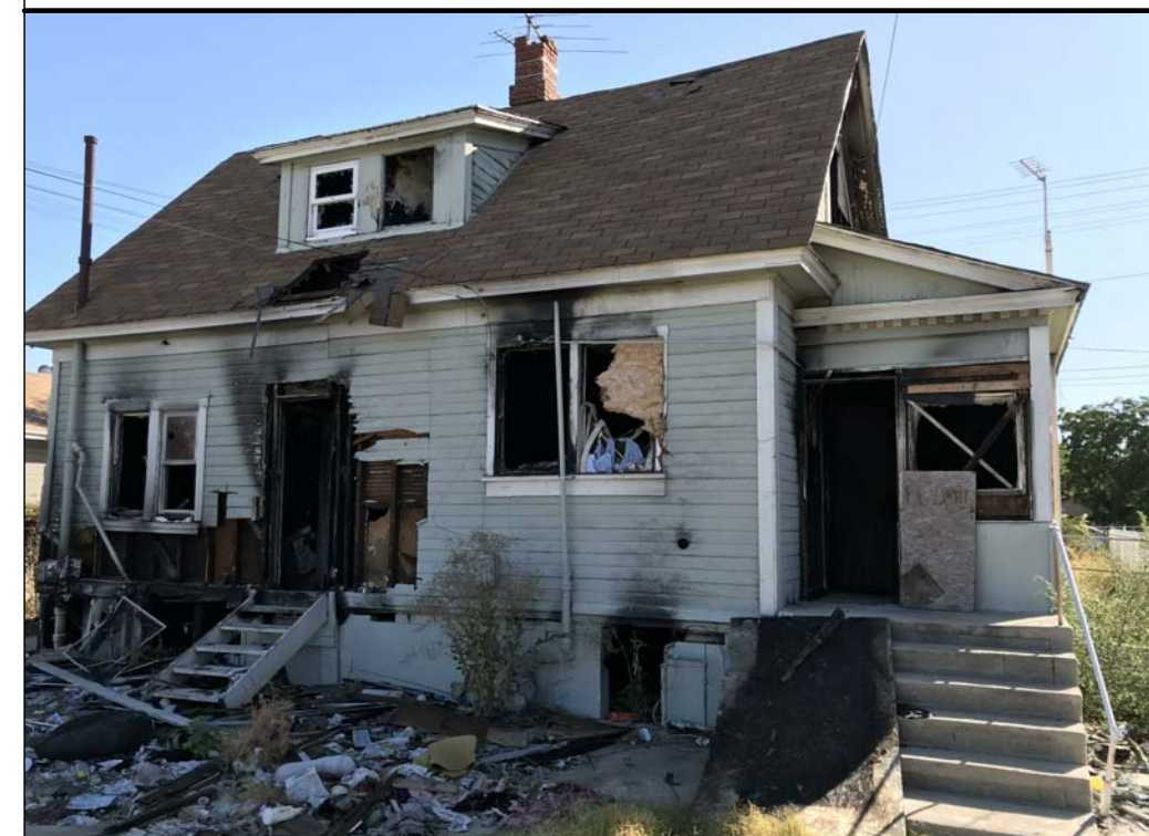
ALL FIRE DAMAGE ELECTRICAL WIRE OR IT DOES NOT MEET CBC 2016 WILL BE REMOVED AND REPLACED
