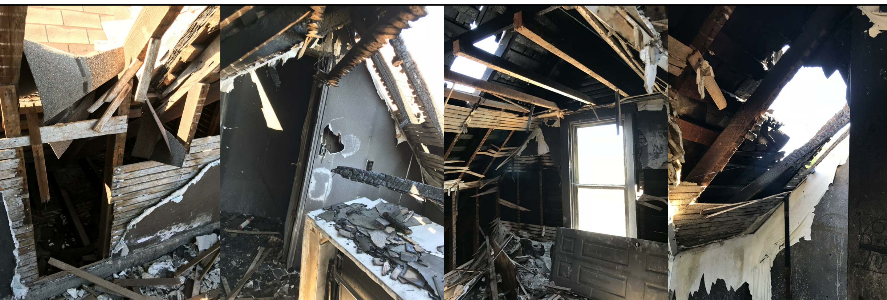
EXISTING FIRE DAMAGE ROOF FRAMING AND SHEATHING TO BE REMOVED AND REPLACE (SEE PROPOSED ROOF PLAN FOR NEW LAYOUT)
