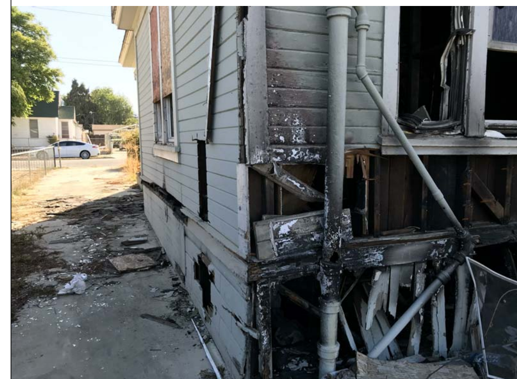
ALL FIRE DAMAGE SEWER OR IT DOES NOT MEET CBC 2016 WILL BE REMOVED AND REPLACED
